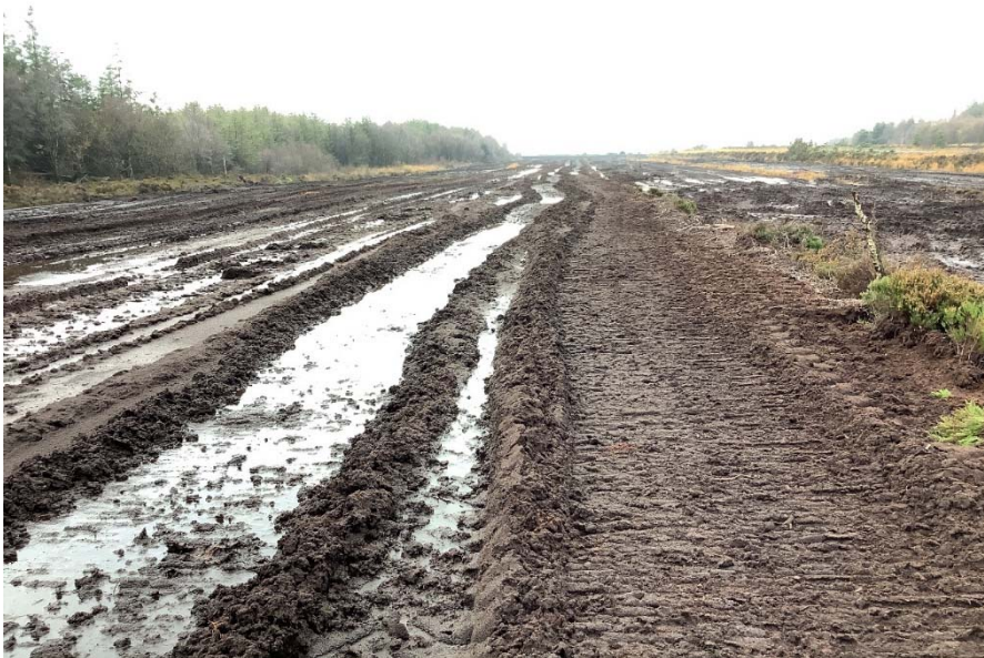
Plate 7: Proposed road from T2 to T3 looking south-west, intersected by bog railway just to north of proposed road.
