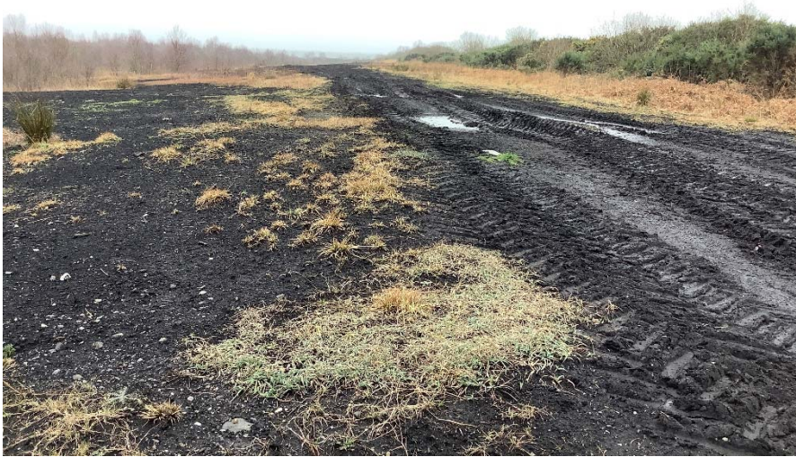
Plate 110: Continuation of proposed road in a southerly direction looking southwest taken from area to northwest of proposed substation site.
